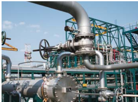
Gas recovery unit
