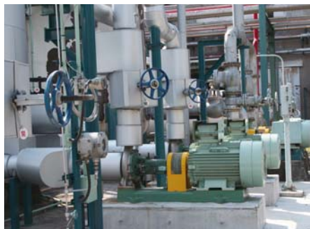
Plant cold water unit
