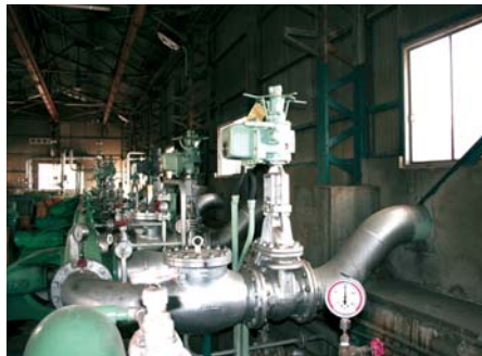
Cooling water supply unit
